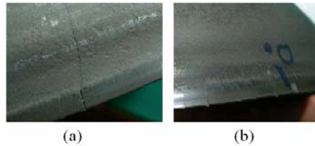
Fig. 6 Surface cracks of shell spun at 760℃
