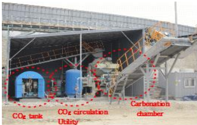
Figure 3. Recycled aggregate pH reducing facility
