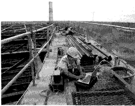
(b) FBG sensor monitoring
