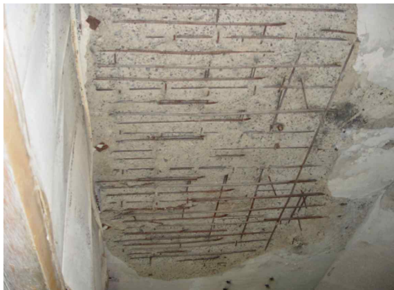
<Fig. 7> Real photography of damaged upper slab
