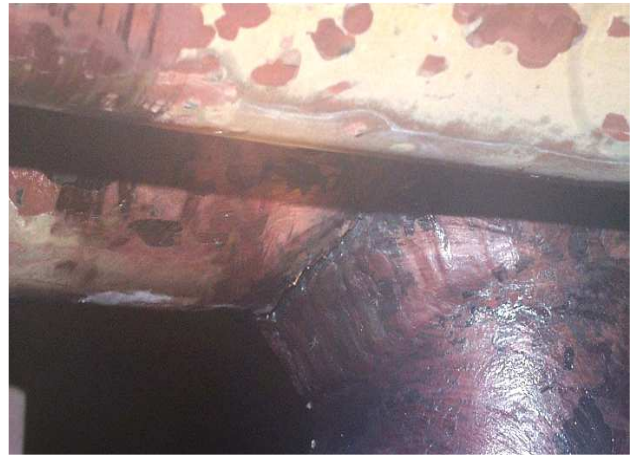
(a) Crack in tube header of cycling unit
