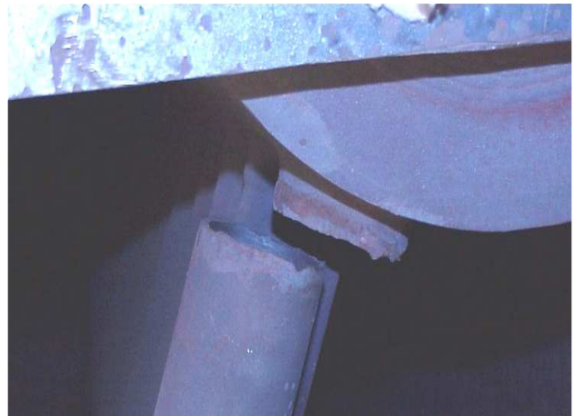
(b) Low cycle fatigue failure of reheater tube
