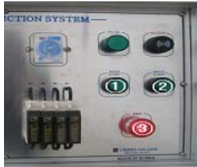
(a) Control panel
