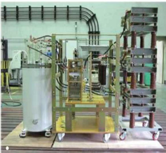
Fig. 1. Hybrid superconducting fault current limiter (KEPRI&LSIS)
