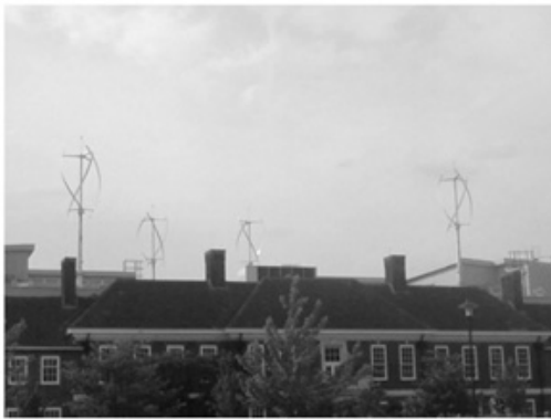
Defra, Weybourne Four turbines installed on a roof top of Defra
