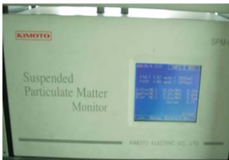
(c) Air-quality monitoring system
