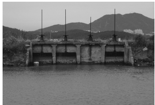
Fig. 3. Experimental water gate located at Dolsan island, Yeosu city (Gate breadth: 10,000mm, Water depth during experiment: 2,500-3,000mm).
