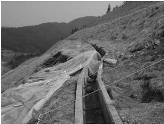
Fig. 5. Failure due to tension cracks (20 months after investigation).
