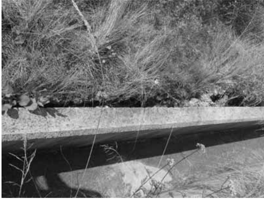
Fig. 4. Observation of tension cracks (July 2007).
