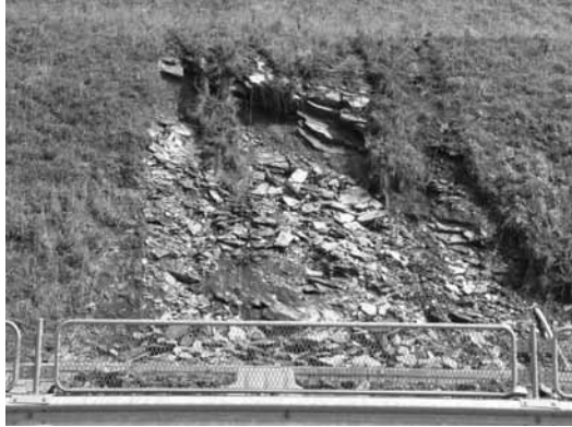
Fig. 9. Failure zone at 136-148m portion of cut slope.
