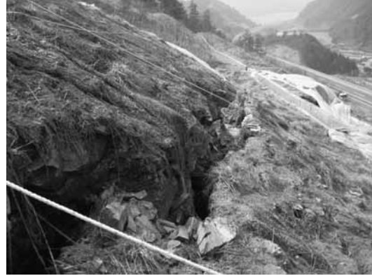
Fig. 7. Expansion of tension crack (20 months after investigation).
