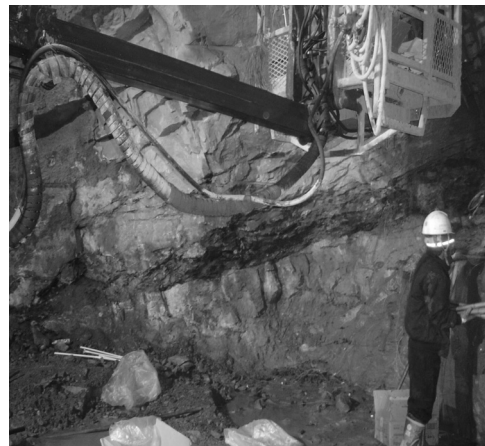
(b) Weak zone at the left wall
