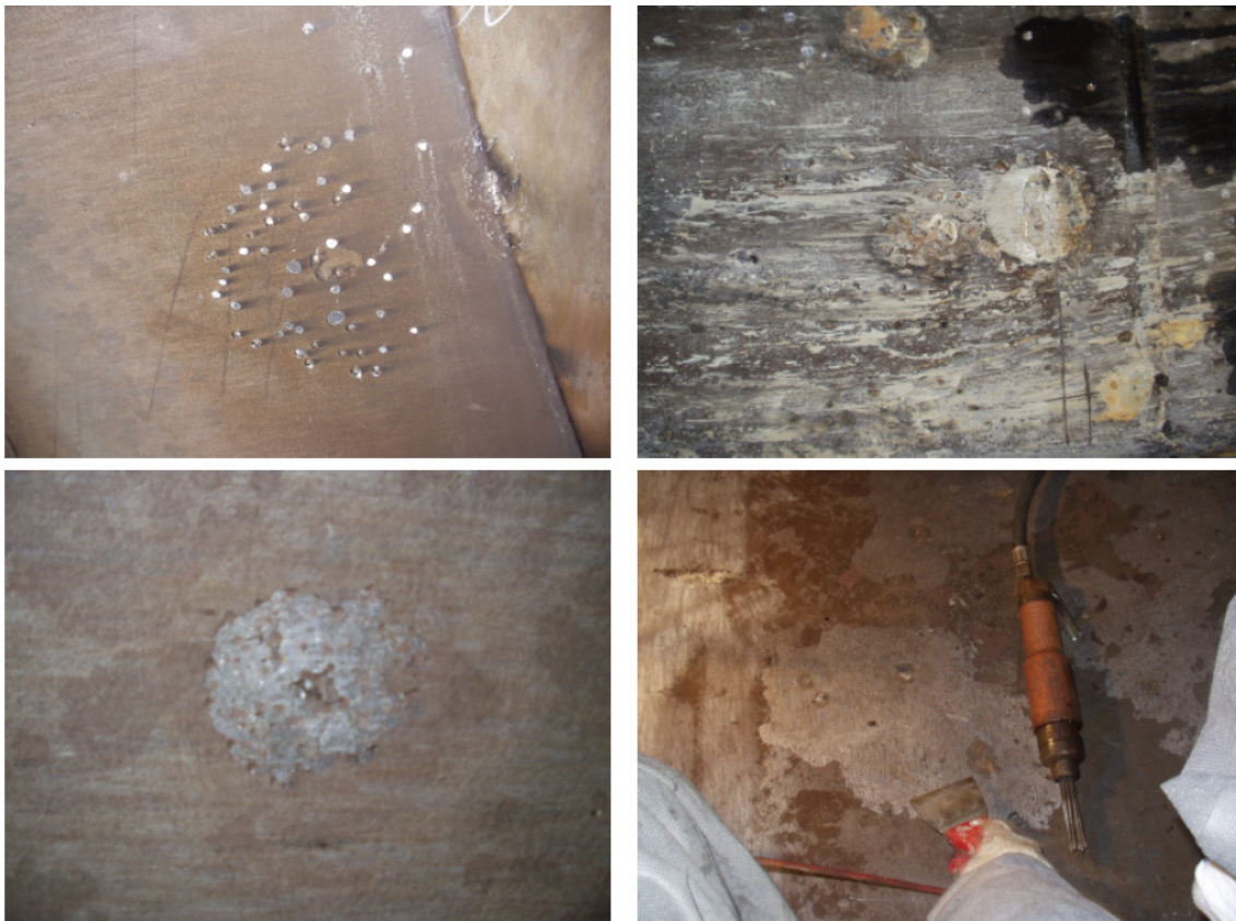
Fig. 4. Localized corrosion propagation after coating failures in seawater pipes.
