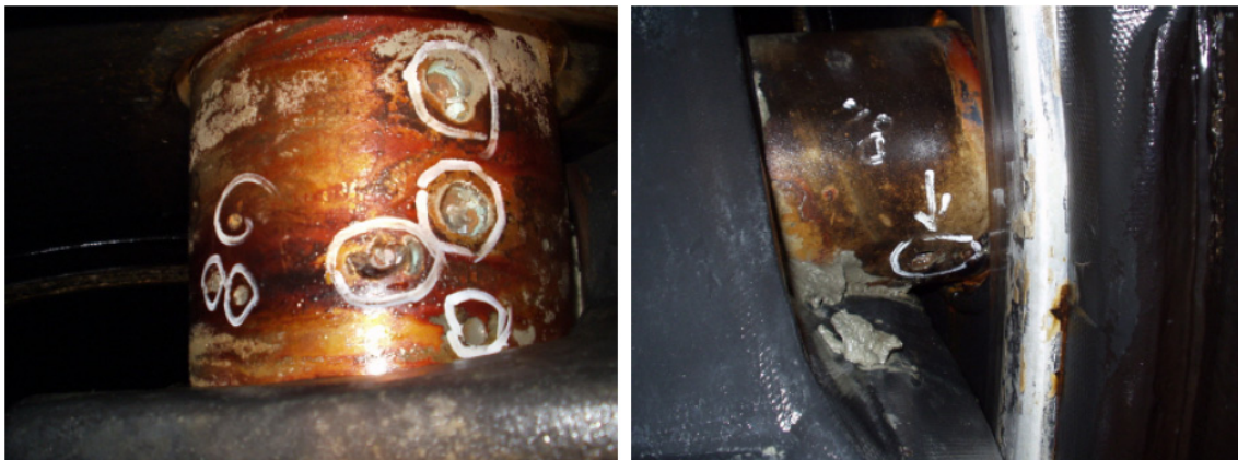
Fig. 5. Localized corrosion damages after rubber liner failures in seawater valves.
