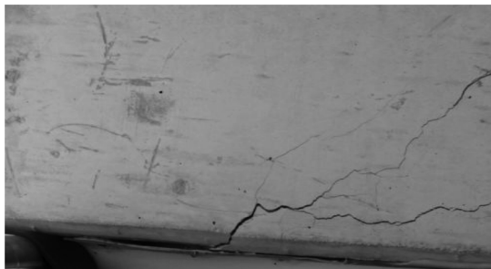
(b) Aspect of Damage 2 – Peeling failure and Concrete Separation
