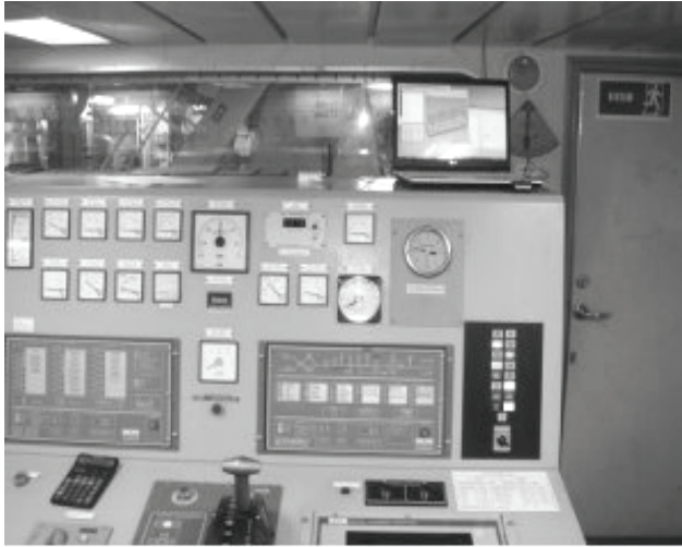
Fig.7 Control room for main-engine operation.
