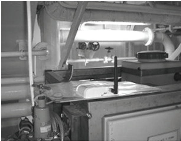
Fig. 8 Router for the WSN in the main-engine room.
