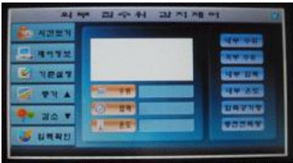
Fig. 5. Flood level detection and control device
