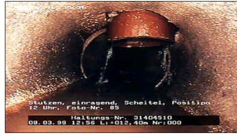
Fig. 3 Protrusion of Connection Pipe
