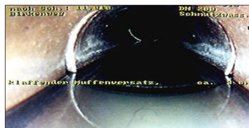
Fig. 6 Bad Connection and Leakage
