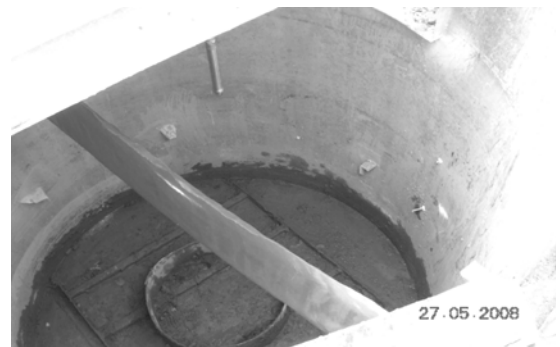
Fig. 3. Internal structure of sediment settling pond.
