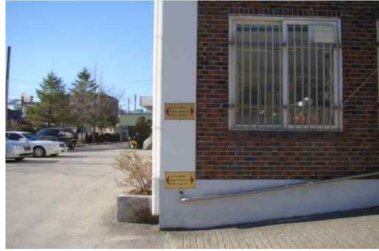
Fig. 4. The Flooding Marks of 2002 and 2003 in Inundated Area (S2)
