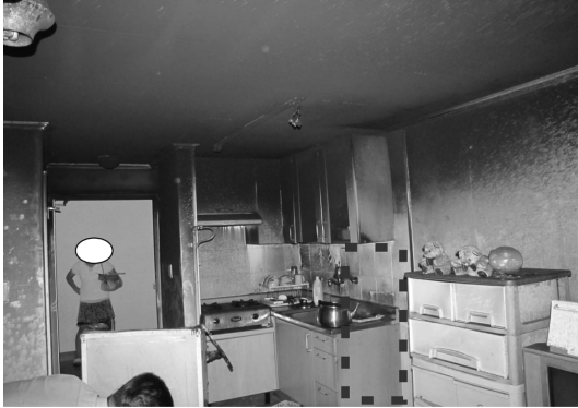
Figure 2. Inner structure of burned house.
