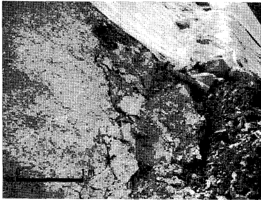
Fig. 5. Settlement of berm.
