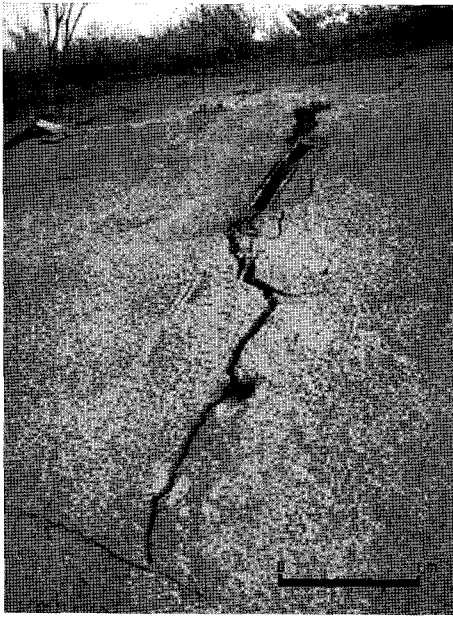
Fig. 4. Vertical crack on shotcrete.
