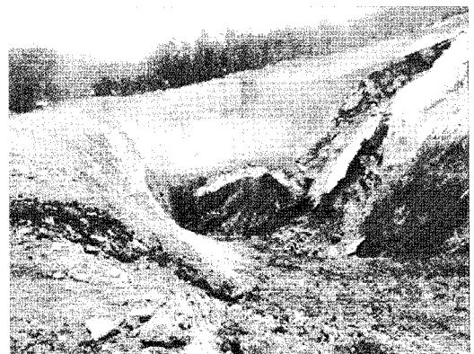
Fig. 2. Collapsed right slope.
