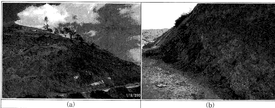
Fig. 1. Quickly weathered slope surface after excavation. (a): Shale at Pasir coal main in Indonesia (b): Shale in Hongjeom Formation at Donghae high-way.
