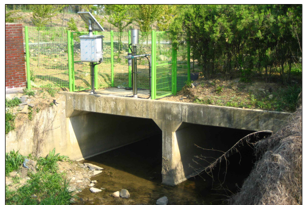
Fig. 4. Outlet Culvert and T/M Equipments
