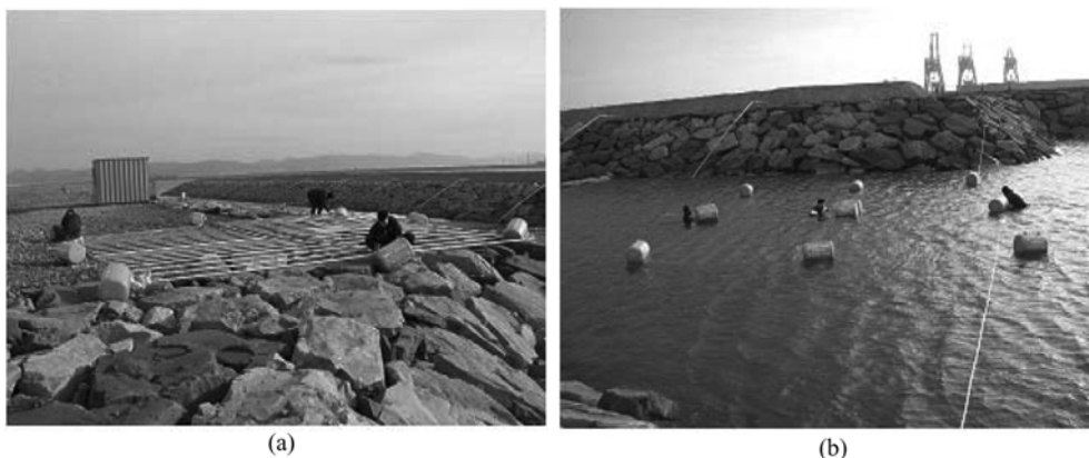
Fig. 4. Photographs of set up steel frames on artificial seaweed beds; (a) construction of steel frames, (b) set up steel frames in the spillway.
