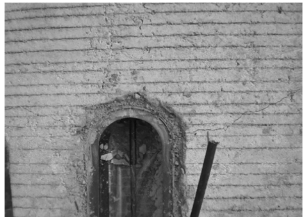
Fig 2. Cracking in pocket.
