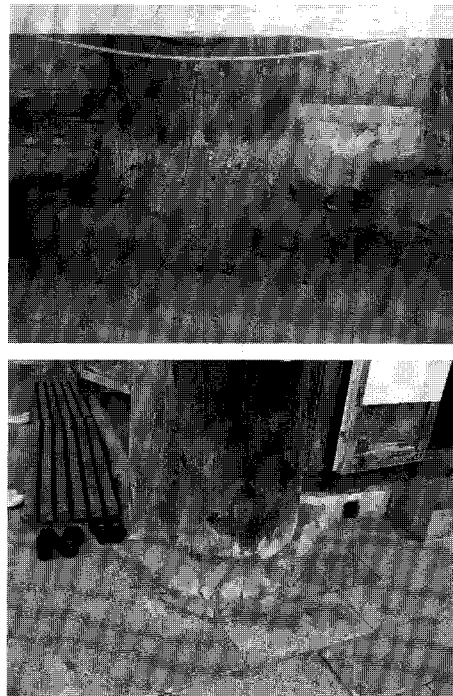
Fig. 4 the state of the bottom of columns
