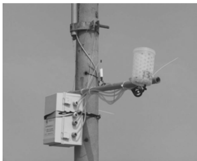
Fig. 4 Universal sample pumps installed in position
