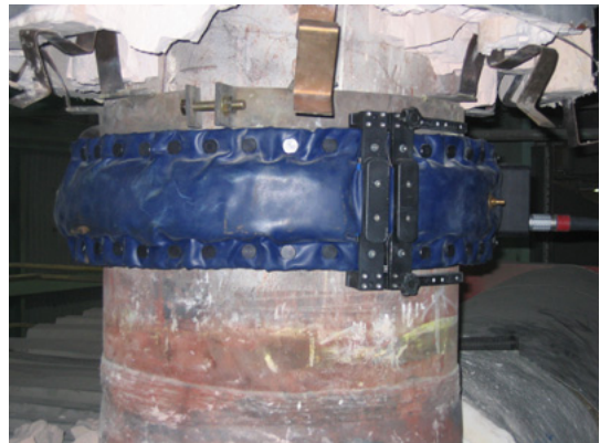
Fig. 14 Photo. of the main steam pipe
