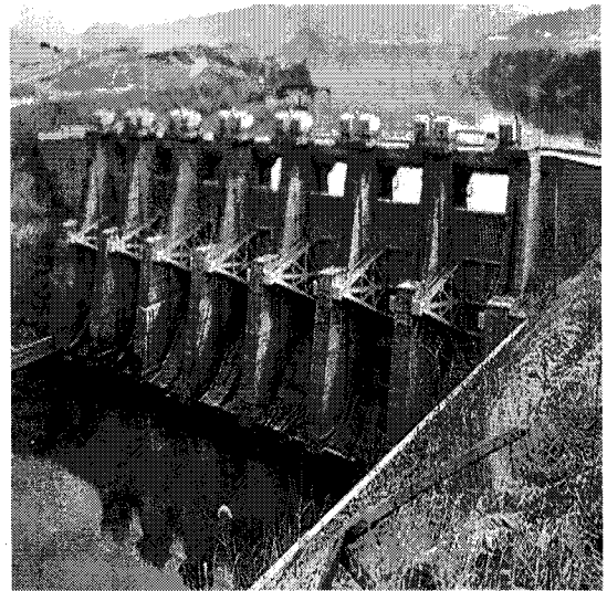
Fig. 2. Yeoncheon Dam(before failure).
