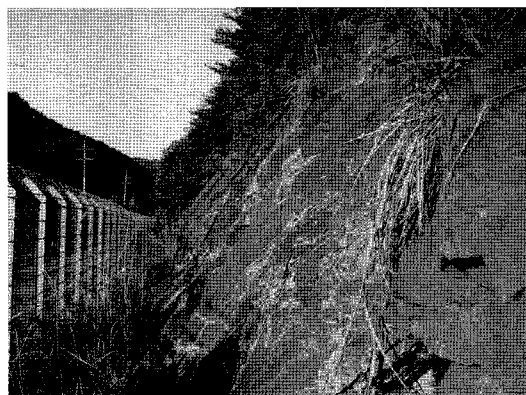
(b) Weathering aspect in site 2
