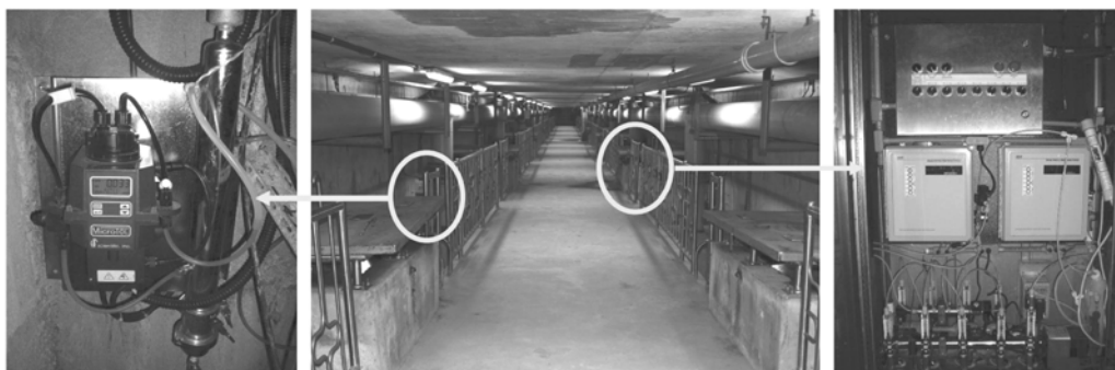
Fig. 2. Turbidity meter (left) and particle counter (right) in filter bed.
