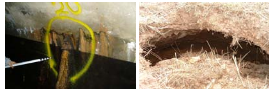
Fig. 3 Damage of water supply dam managed by local governments (a) Loss and solidity of core material through the concrete lining, (b) Sinkhole in the dam crest
