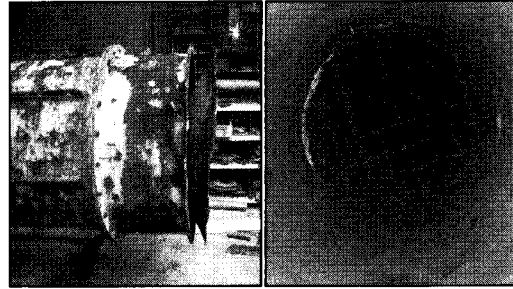
Fig. 6. Throttle valve(left) and steady flow unit(right).
