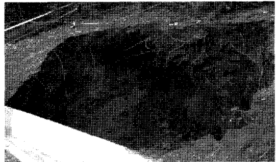
Fig. 8. “A” tunnel collapse shape.
