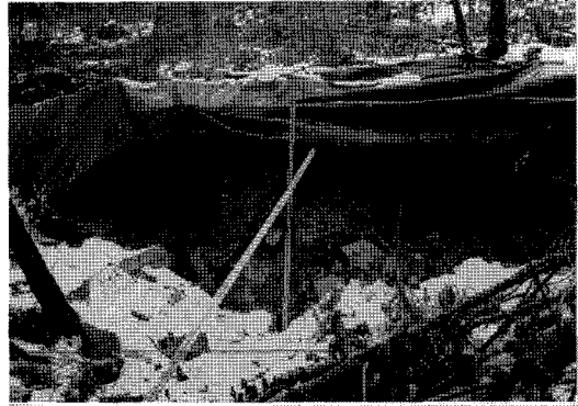
(b) ④ width 0.4m / differential settlement 2.0m strike, dip : N59W, 87NE
