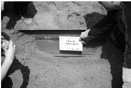
Fig. 3. Status of sand compaction condition by watering at lower part of bottom pipe line
