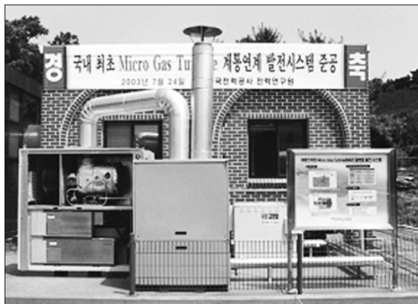
Fig. 1 60kW class Micro Gas Turbine(MGT) Co-generation system (Korea Electric Power Corporation) - Capstone Turbine Corp. C60 mode
