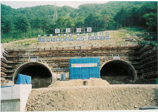
Photo 1. View of inlet zone
