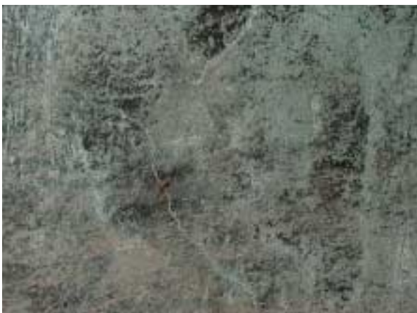
Photo. 9. Internal view of the cracks
