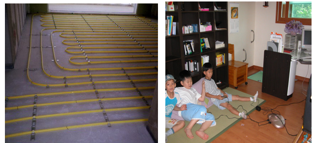
Picture 5. Panel heating system
