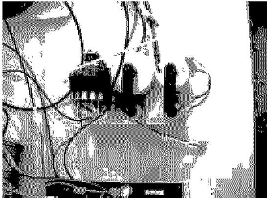
Fig. 14. The high voltage transformers.
