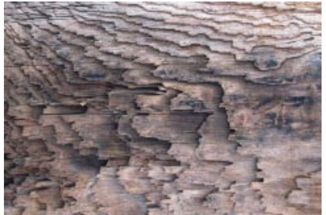
Fig. 8. As weathering continues, erosion takes place.
