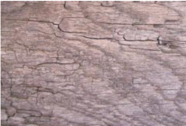
Fig. 7. Cracks were caused by moisture observed at the surface wood tissues.
