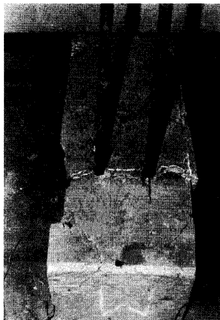
(a) Radial Cracks
