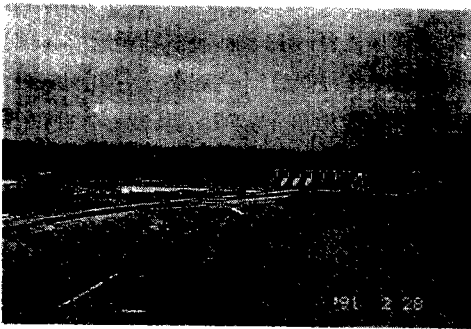
Fig. 8. Down stream of karasaan weir left side is sand trap construction/Right site is by pass water way
