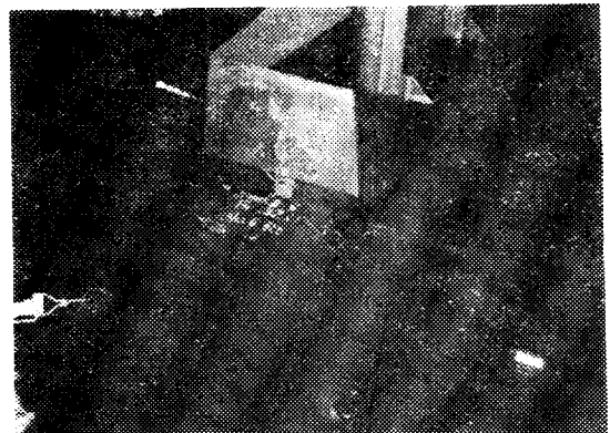
Proto 2.3.2 Partial bulkhead corner on No.6 deck at Fr.132(S1 in Fig.2.3.1)
