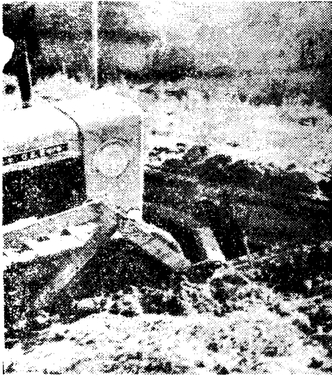
Fig. 2. Dozer is pushing soil to angled direction by turning at the forward working method
