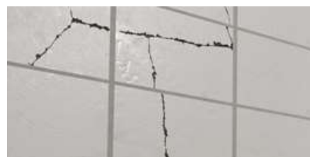
Figure 2b. Tile with defects
