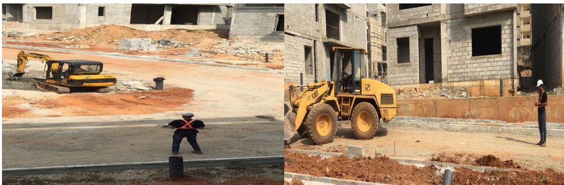
Figure 3. Sound detection experiments with a front-end loader (left) and an excavator (right)
