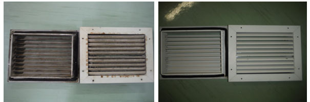
Fig. 2. Photos of grille before and after cleaning.
