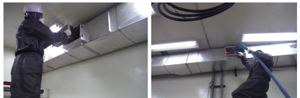
Fig. 3. Photos of grille detachment and duct cleaning.
