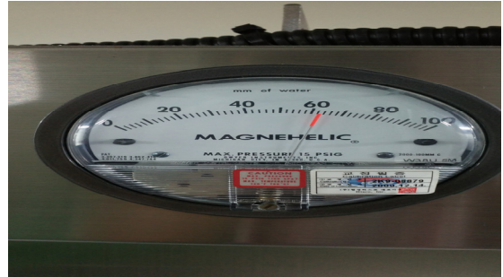
Fig. 2. Differential Pressure Gauge(HEPA).
